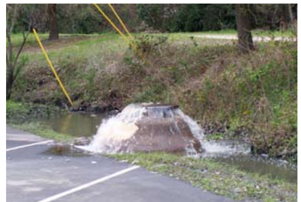
Inadequate tunnel capacity causes sewer overflows
