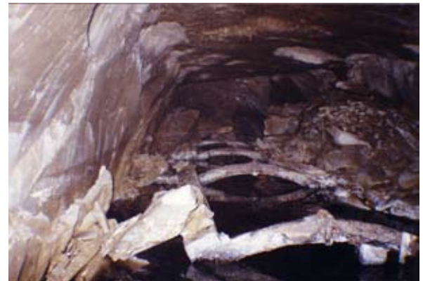
This photo taken by divers inspecting the tunnel shows complete collapse of the tunnel structure. This section of tunnel has been replaced.
